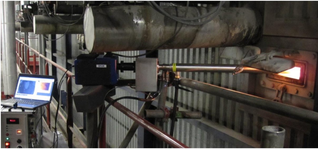
Figure 7 Inspection of flame during adjustment of burner settings (swirl) with combined VIS and IR endoscope system inserted into boiler. Pyroptic offer mobile and permanent installed systems.
