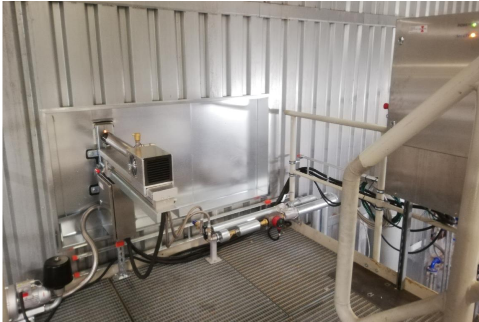
Figure 8 IR camera system with two thermal cameras built into a water-cooled probe. Installation from straw and wood fired grate fired boiler at Fjernvarme Fyn A/S, Denmark. The system is controlled from the control room and images of the burning biomass displayed in Milestone.
