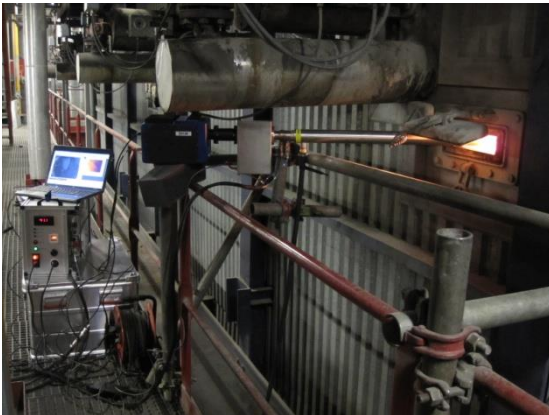
Portable combined video and IR imaging system for boilers using evaporation cooling (5-10 liter water per hour).
